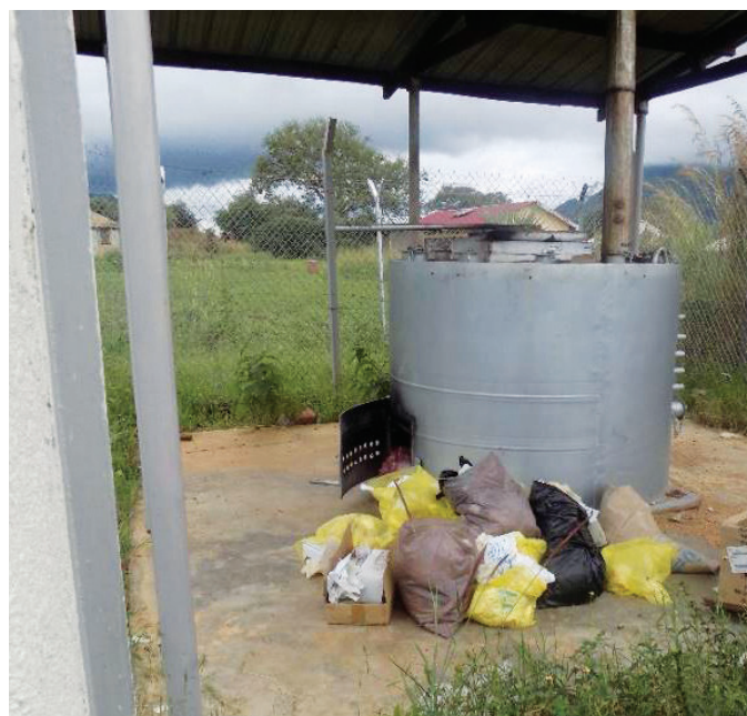
Incinerator at Alerek HC III
