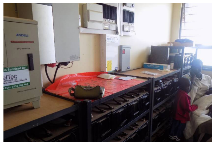
Solar System in Abim General Hospital
