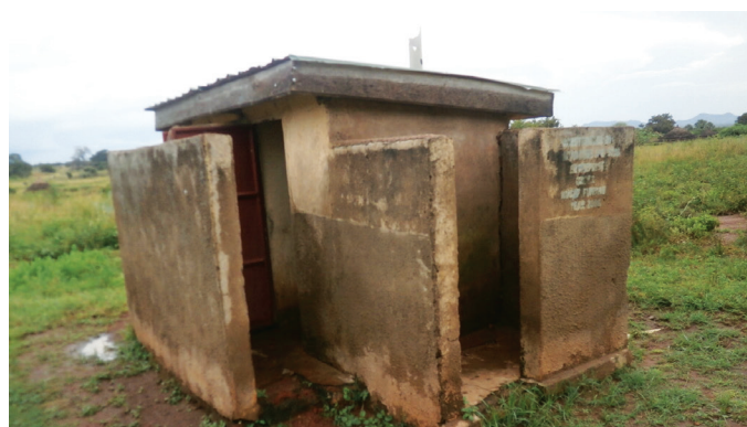
Latrine in Obolokome HC II
