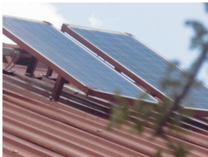
Solar pannels at Alakas HC II
