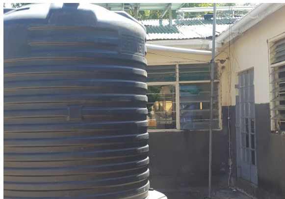
Water storage tank in Nabilatuk HC IV
