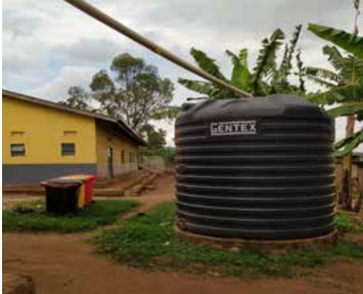
Water harvesting at Ngarama HC III
