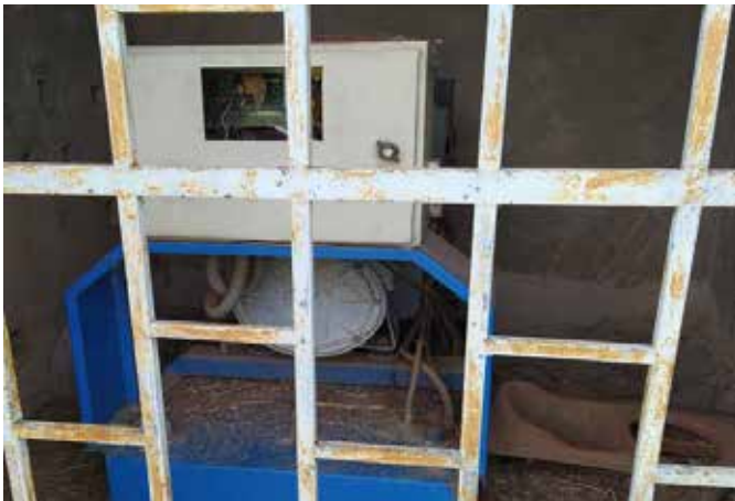
Non functional generator at Nyamuyanja HCIV
