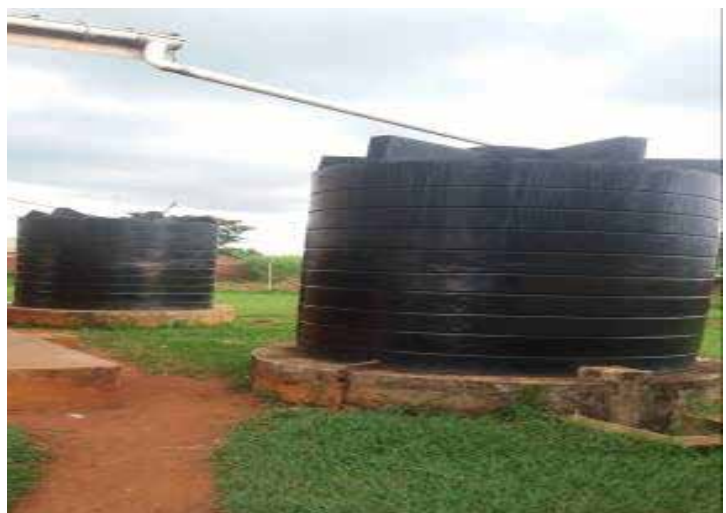
Water tanks at Kitayunjwa HCIII
