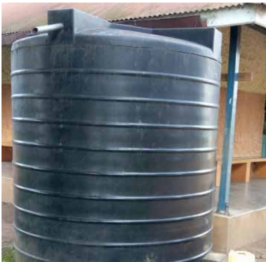
Water tank at Namasagali HC III
