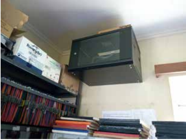
Server room and ART records that are securely locked to keep confidentiality
