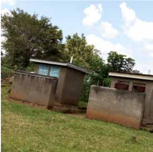
Toilets at Namasagali HCIII
